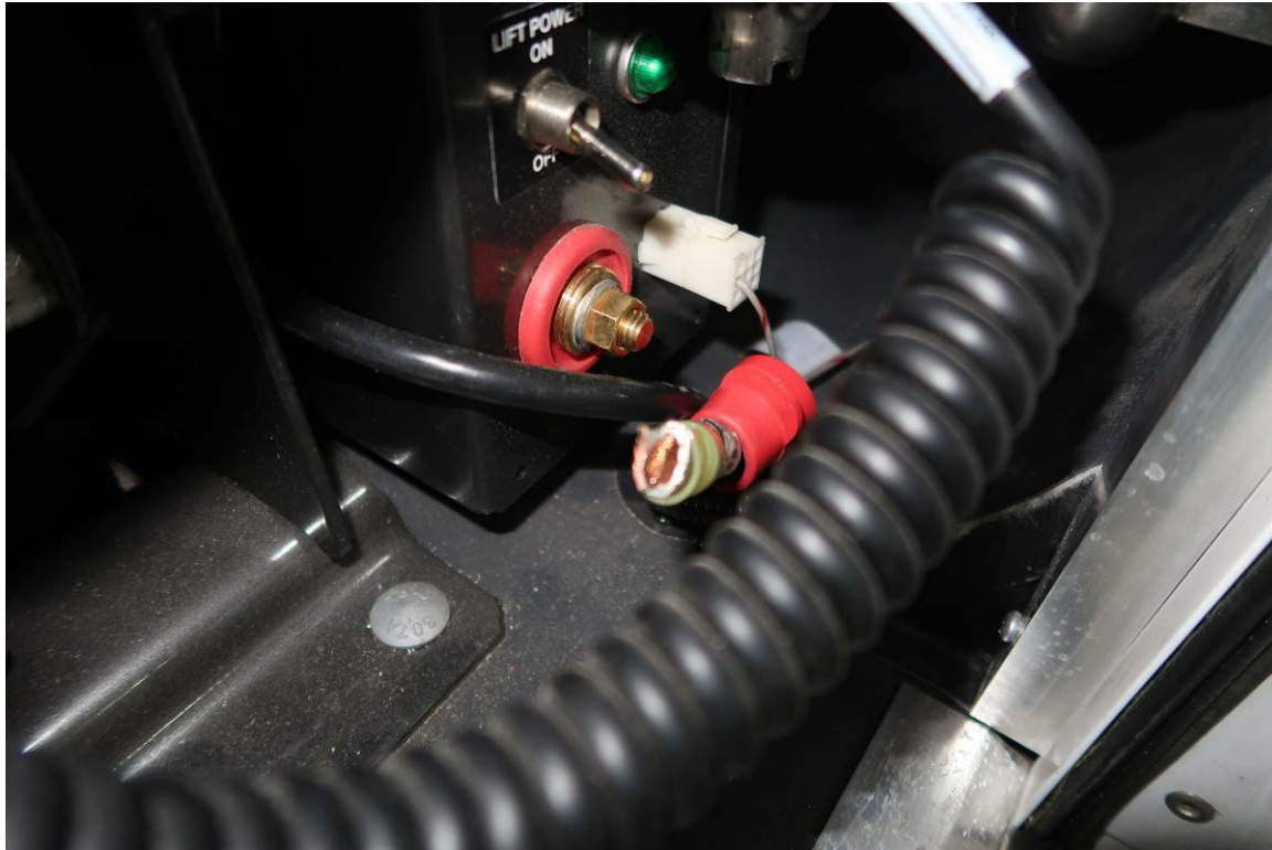
12-VOLT POWER SUPPLY CABLE BROKE AT THE ADA LIFT (2,766 TEST MILES)
