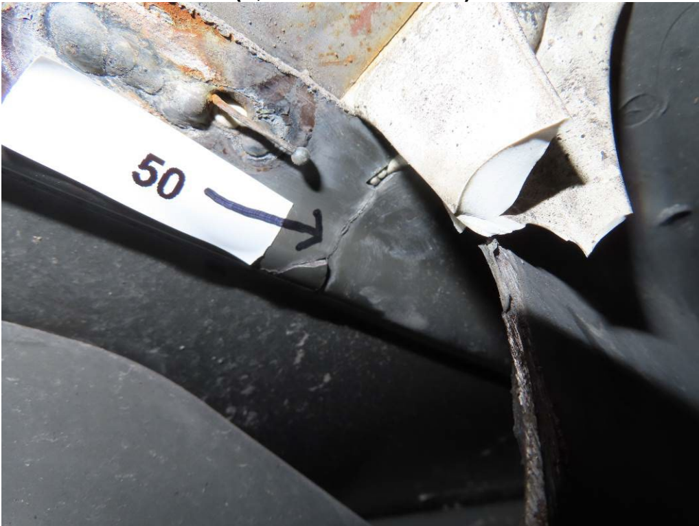
CRACK #50– BODY ABOVE FRAME RAIL BETWEEN BODY MOUNTS BEHIND CURBSIDE FRONT TIRE (7,486 TEST MILES)
