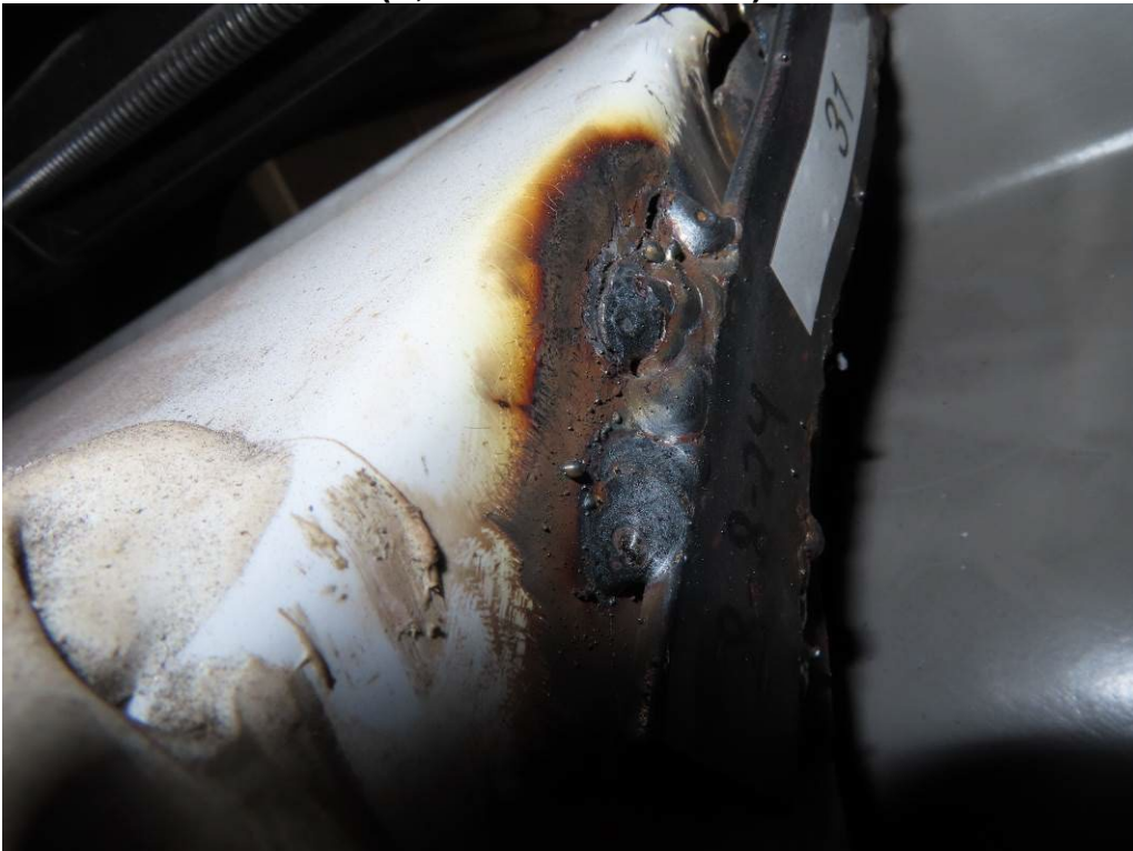
CRACK #31-2– PREVIOUSLY REPAIRED SUPPORT GUSSET ABOVE DRIVER'S DOOR CRACKED AGAIN (7,486 TEST MILES)
