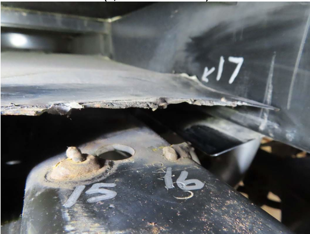
CRACKS #15, 16 & 17 – ADDITIONAL CRACKS WHERE HEATSHIELD WELDED AT THE REAR (1,123 TEST MILES)
