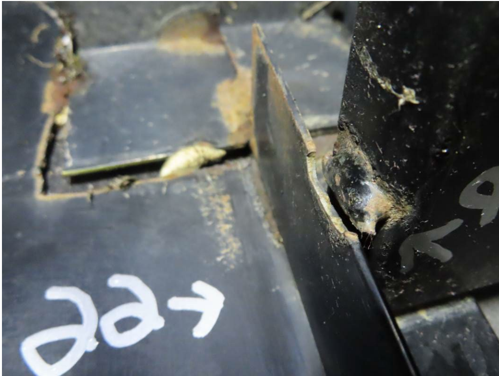
CRACK #22 –BROKEN WELD ON CROSSBEAM IN FRONT OF STREET-SIDE REAR TIRES WHERE IT ATTACHES TO SUPPORTING FRAMEWORK (1,123 TEST MILES)
