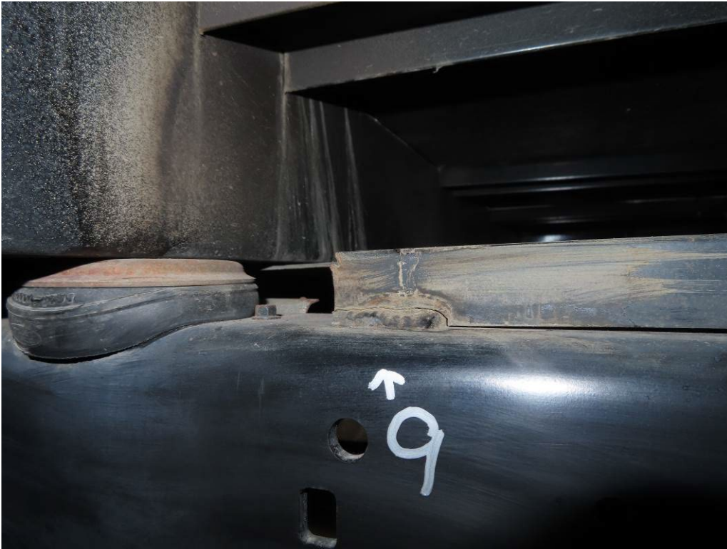
CRACK #9 – TOP OF THE CURBSIDE FRAME WHERE THE HEATSHIELD IS WELDED (1,123 TEST MILES)
