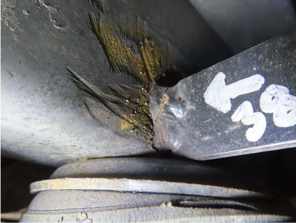
CRACK #38 –CURBSIDE HEATSHIELD, WELD IS BROKEN (6,207 TEST MILES)
